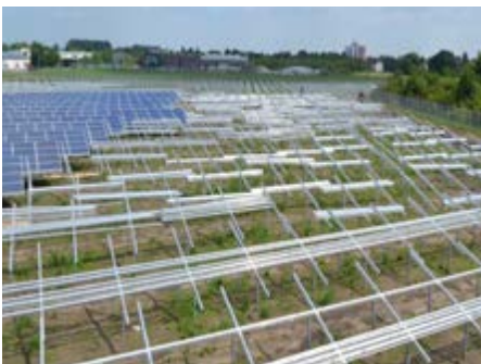
3500 kWp in Nienburg / Hannover, Germany
