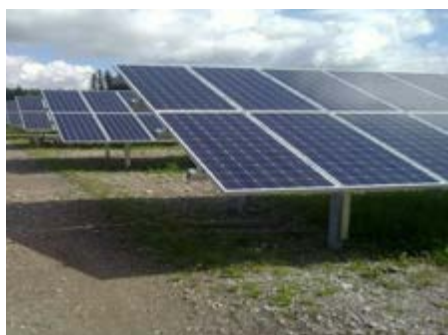
1500 kWp in Türkheim, Germany
