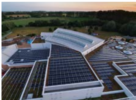
712 kWp rooftop in Stralsund, Germany
