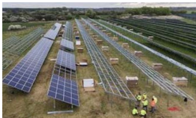
Digging of cable trenches and the relevant foundation work for the transformer stations.
