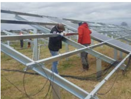
750 kWp in Pakendorf, Germany
