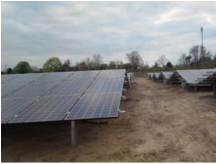
3150 kWp in Coburg, Germany
