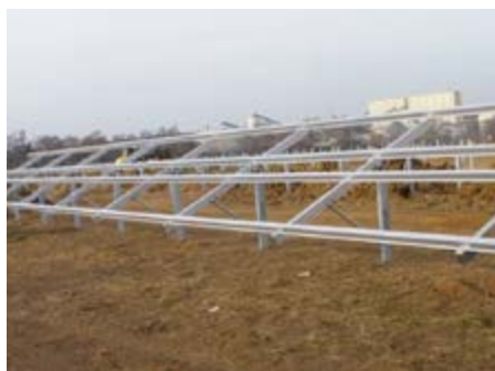
1500 kWp Leipzig, Germany
